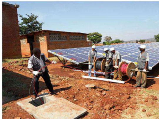
Fig. 14.15 Installing a hybrid solar power system at the DREAM center and laboratory. Mhengo wa Ntenga (Lilongwe) Malawi
