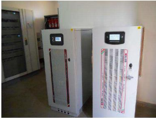
Fig. 14.3 AROS SPS hybrid solar inverters powering DREAM center and laboratory. Balaka,
